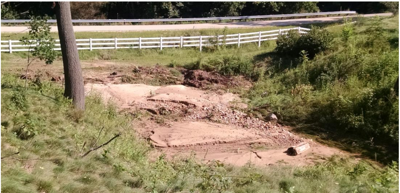
Sediment and debris closed the drainage system from the ravine along Blackhawk Rd.
