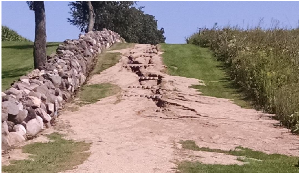
Screened trail damage
