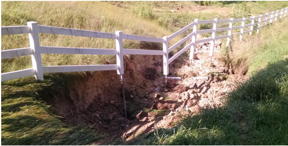
Erosion along Blackhawk Road
