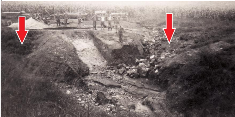
Above: 1938 photo of CCC construction of spillway. Note the erosion taking place at the sides of the spillway.
