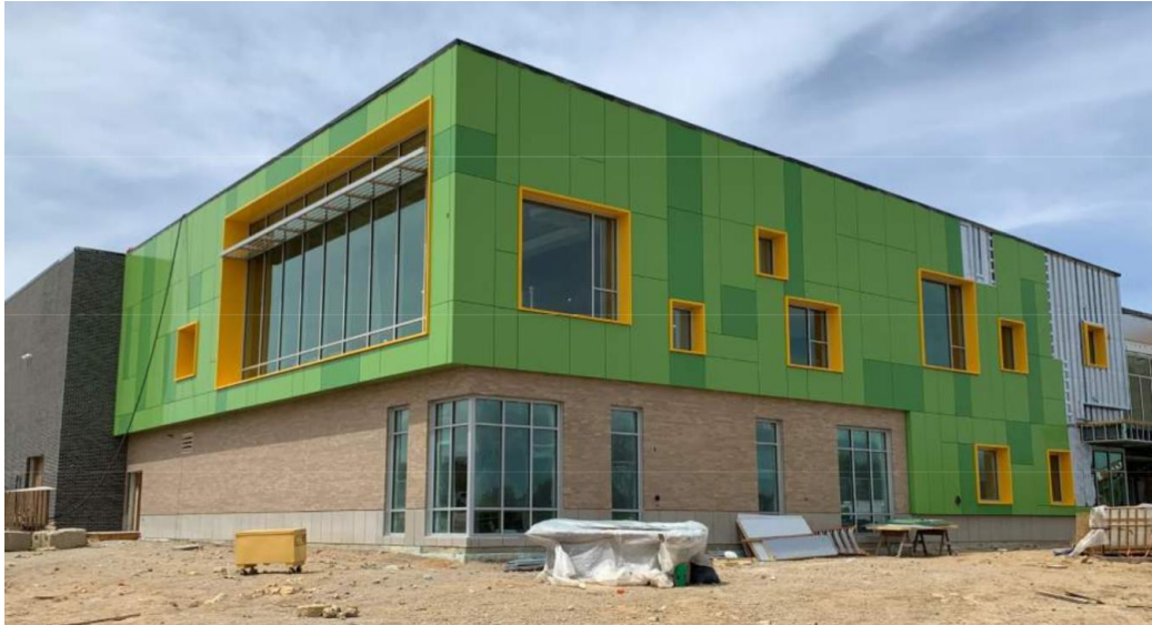
Above: Exterior metal panel progress on the southeast side. The south side is completely finished with green panels, while the east side nears completion.
