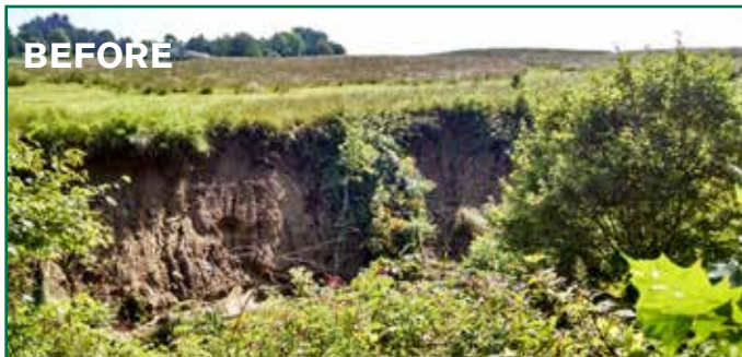
Eroded slope near bottom of ravine after the 2018 storm.
