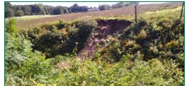
Eroded slope near top of ravine after the 2018 storm.
