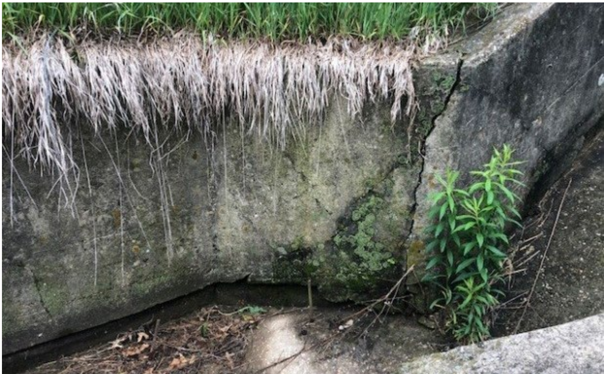
Cracks are visible in the concrete structure at the bottom of the slope. Photo by Jim Bolitho.
